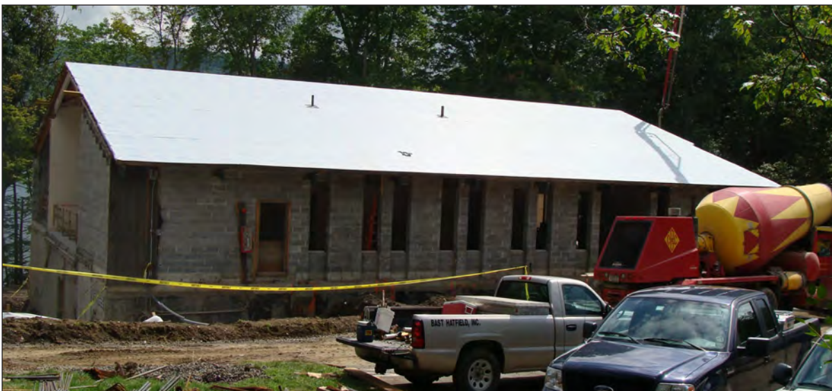
BFS and CGP building as it looked while under renovation on August 24 of this year. Photo compliments of Assistant Professor Michael Flinton, CGP.
